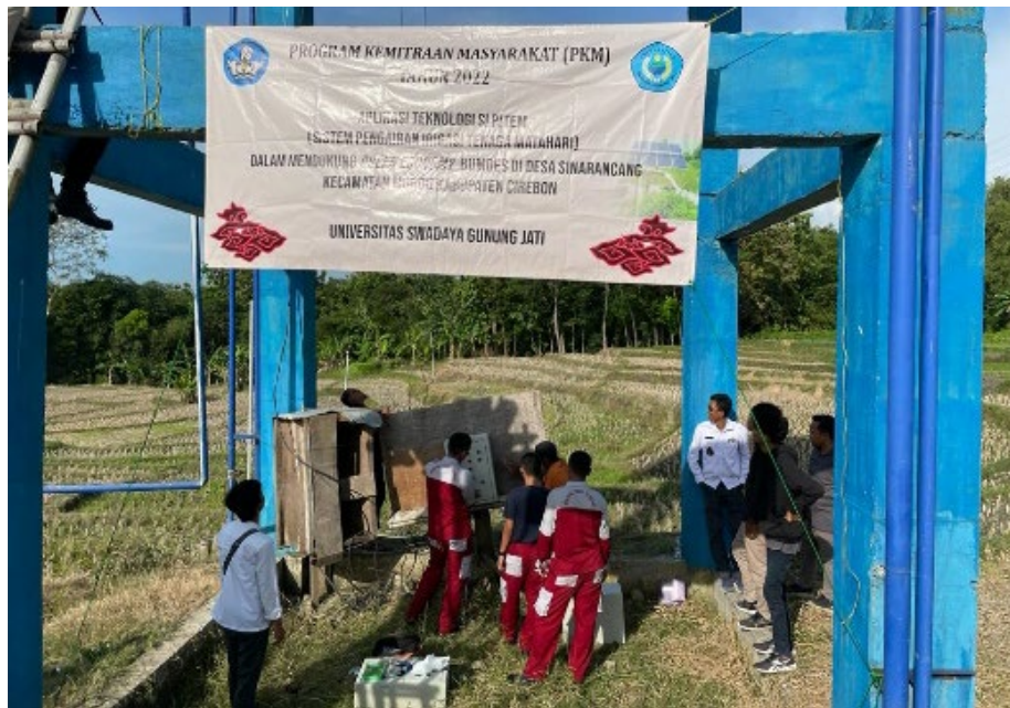
Figure 6. Box controller installation location
